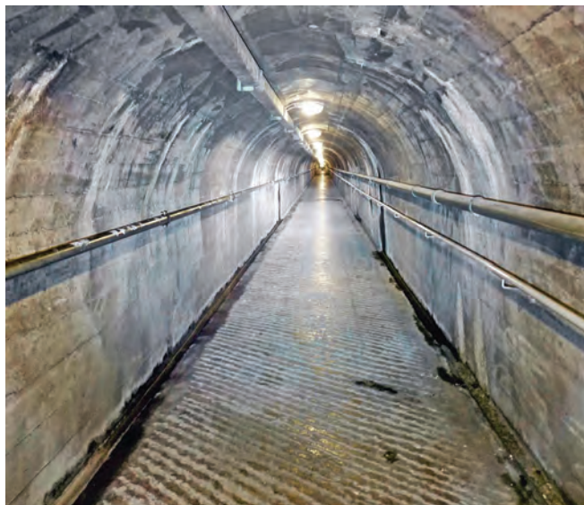
Fort Magletsch: The ramp leading from the turntable chamber to the upper level of the fort
